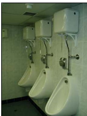
Wall hung urinals with pull chain cisterns
